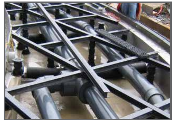
This fountain in Dallas required detailed fabrication of grating and structural components that could be submerged in water without corrosion or rust.
