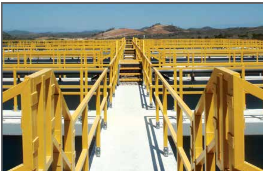
A partial view of miles of railing fabricated for a wastewater treatment facility in Mexico. This project also included several crossover platforms with stairways.
