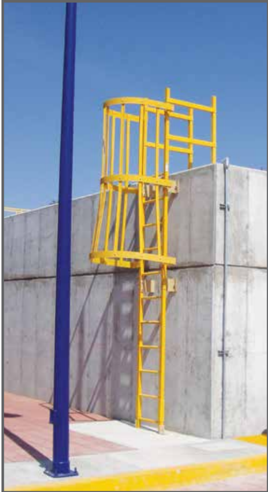
This Dynarail® caged ladder provides safe access for workers at this water treatment facility.
