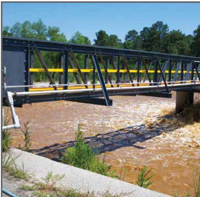
This all FRP truss walkway was designed and engineered to replace an existing rusted steel structure.
