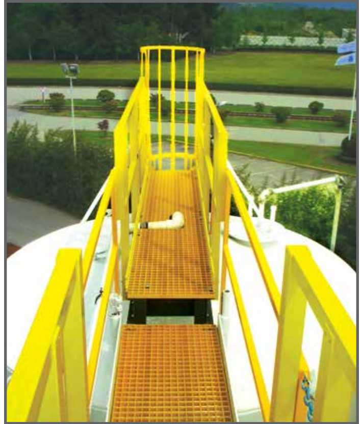
Fibergrate's grating, railings and structure create walkways for worker access to multiple tanks.
