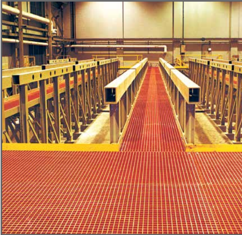
This battery plating facility's demanding corrosive environment required FRP elevated walkways, fabricated from Dynaform® vinyl ester structural shapes and Vi-Corr® molded grating.
