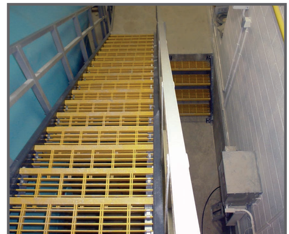
The stairway above utilizes Fibertred molded stair treads to provide tank access at a pumping station.
